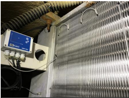
For a DX system ice will built up on the pipes and fins close to the expansion valve. If the superheat pipes on the air inlet side, you can see limited ice built up.
