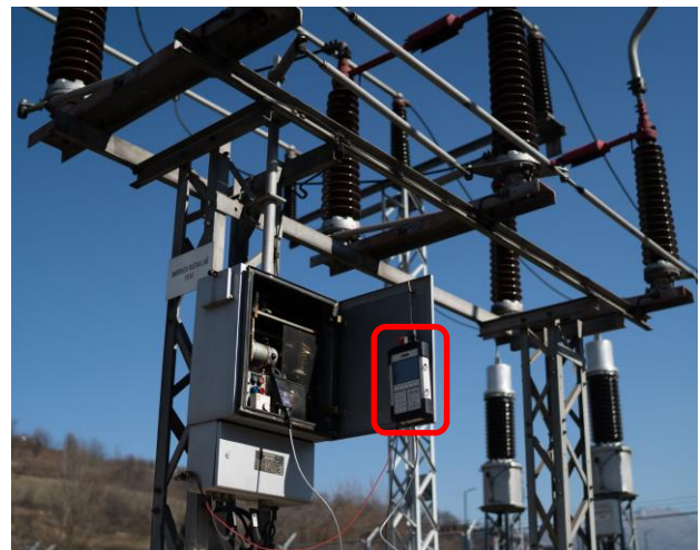
DIS-H mounted on the disconnector's cubicle during testing
